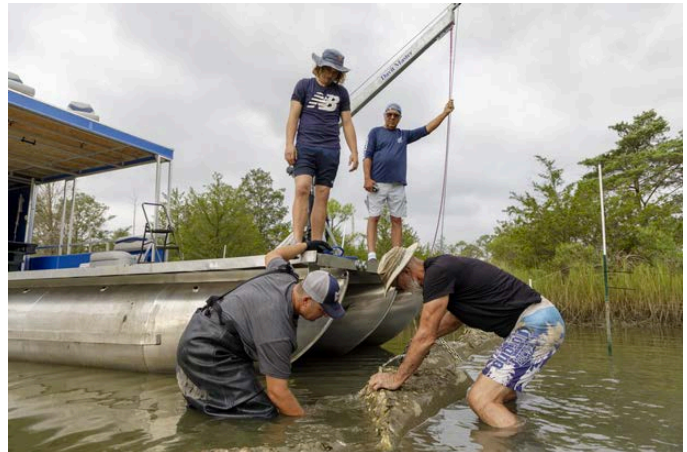
Workers from marine companies that focus on coastal resilience are installing oyster habitat, called oyster castles, made of oyster shells and concrete in a channel of Whittaker Creek in Gloucester, Virginia, to support healthy oysters on Aug 15, 2023. (Photo by Lathan Goumas | Virginia Sea Grant)
